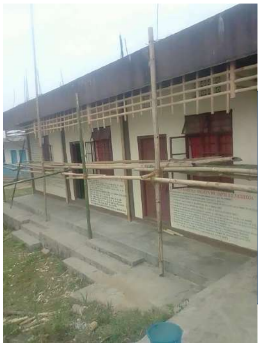
Out of 26 community halls, 11 are undergoing construction, the remaining constructions are on hold due to the lockdown. April 2021; Photos by K. Wahlang, NESFAS
